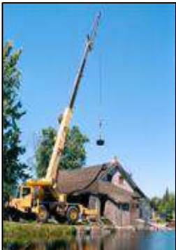
One of the refurbished turbines being put in place by a crane.
